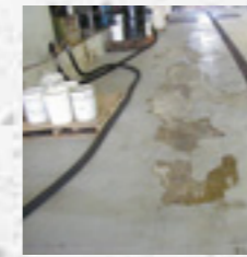
Failed epoxy flooring due to excessive water vapour transmission.
